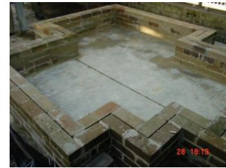
Basic bricked up area on concrete slab to be used as a water feature.
